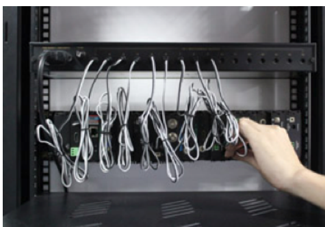
5. Centralise Power Supply installation.
